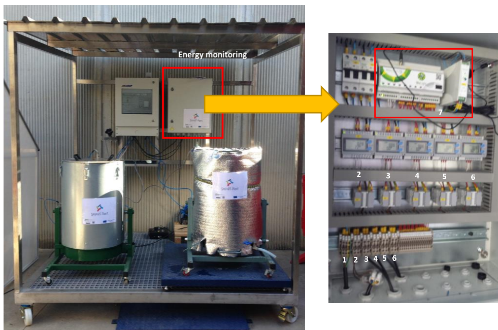
Figure 28 Image of the energy monitoring system.
